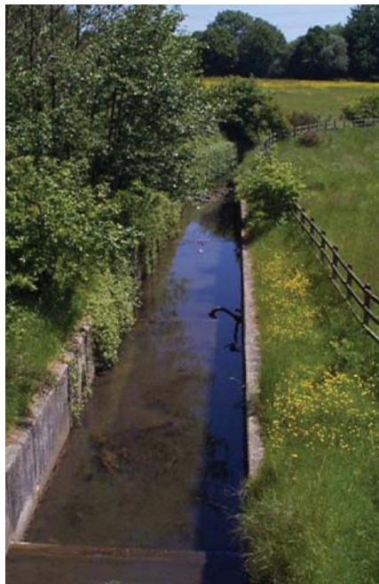
← Concrete lined channels are typical in South East Hampshire. Work is ongoing to restore more natural watercourses.
