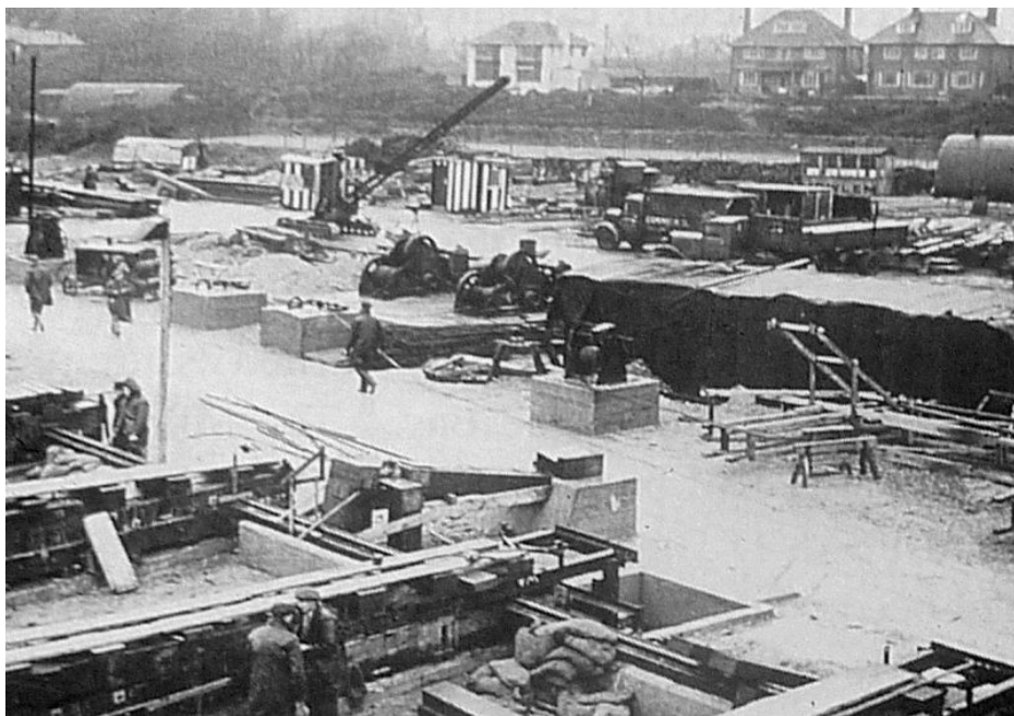
A slipway under construction at the western Phoenix construction site at Stokes Bay (fortgilkicker.co.uk).
