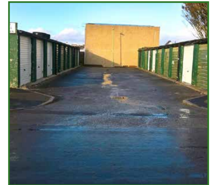
Garages at Dolphin Crescent in need of decoration and repair
